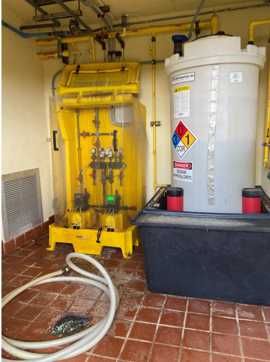
Figure 6. Chlorine Room with Hypo Pumping Skid and Hypo Tank
