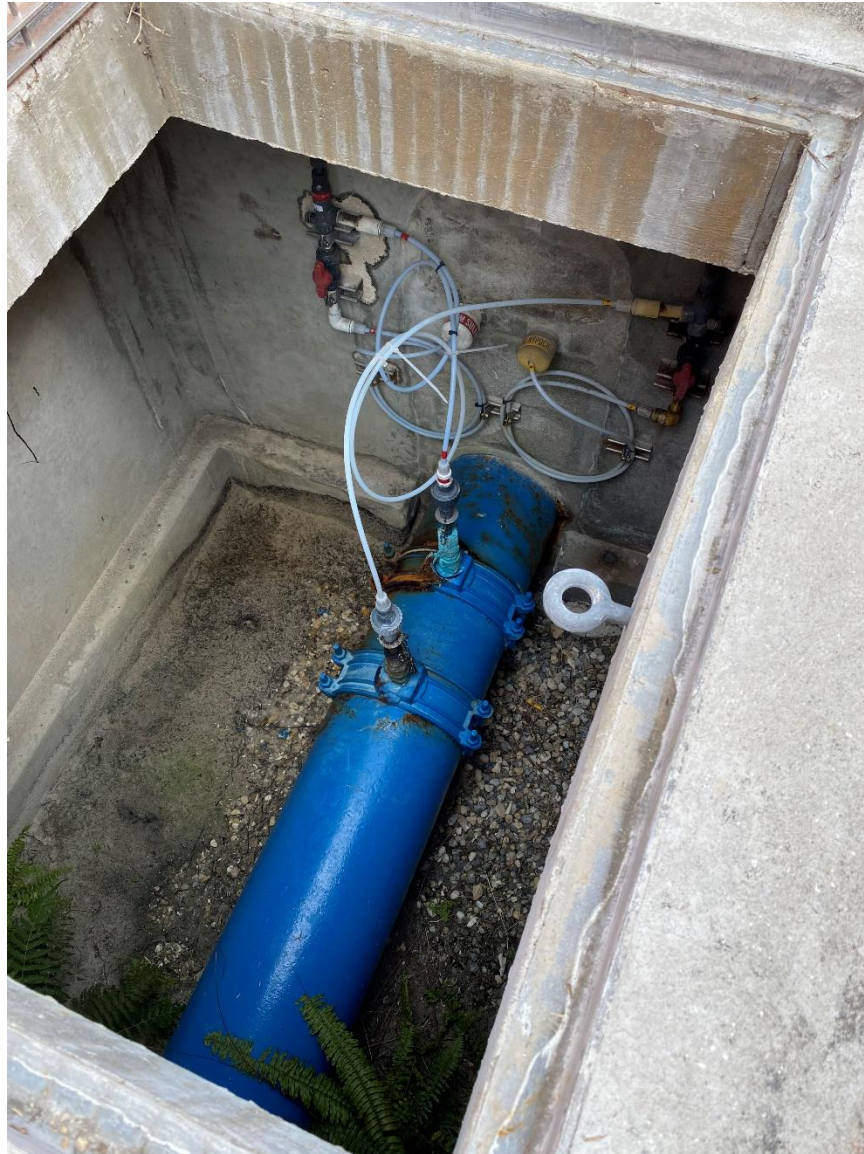
Figure 2. Chemical Injection Vault
