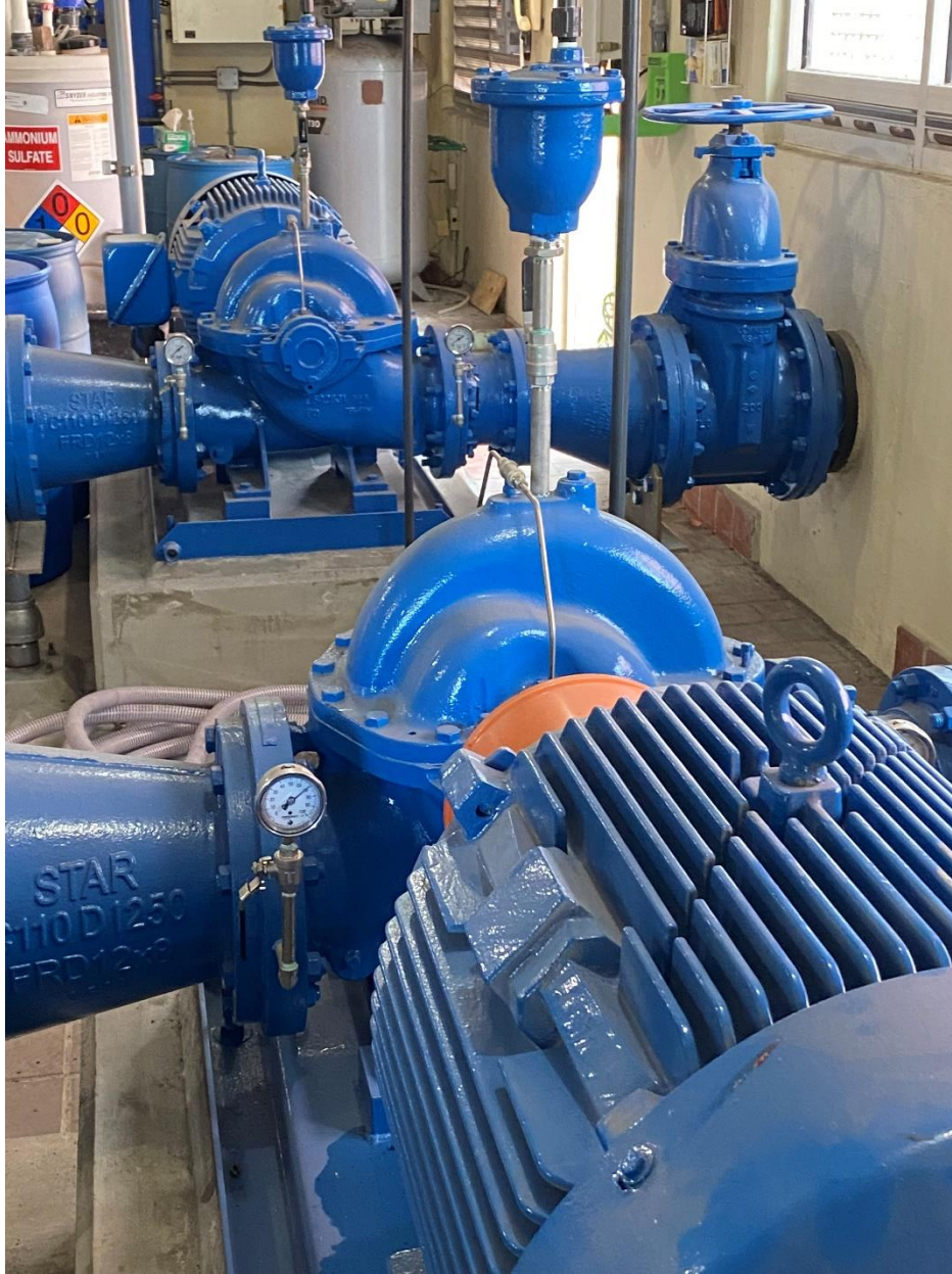
Figure 9. High Service Pumping Area
