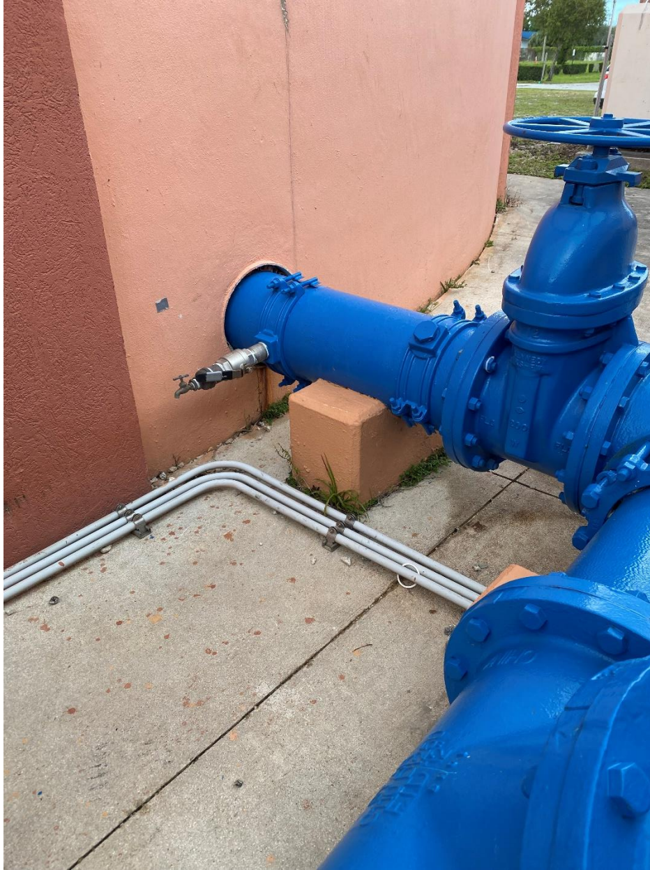
Figure 4. 12" Ductile Iron Pipe Watermain. Note: The water sample for total chlorine residual (4.4 mg/L) was collected from the discharge of the tank here.
