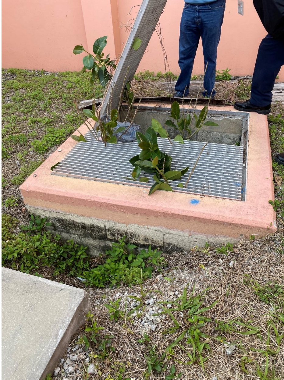
Figure 8. Vegetation Growth in the Tank Drain Vault
