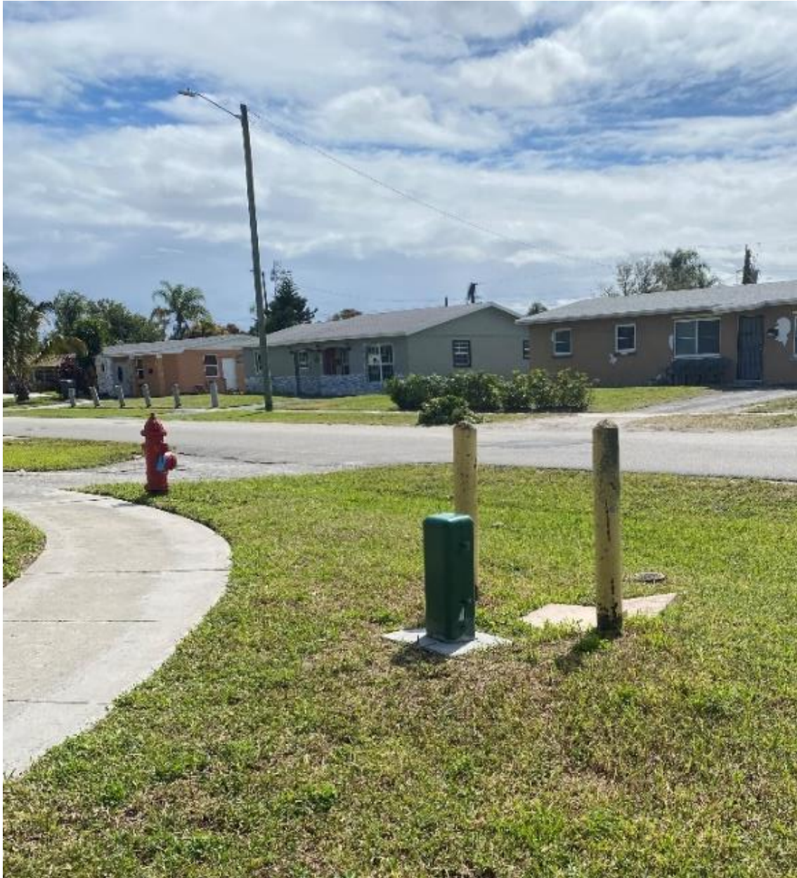
Figure 4. Proximity of SP #38 to Fire Hydrant
