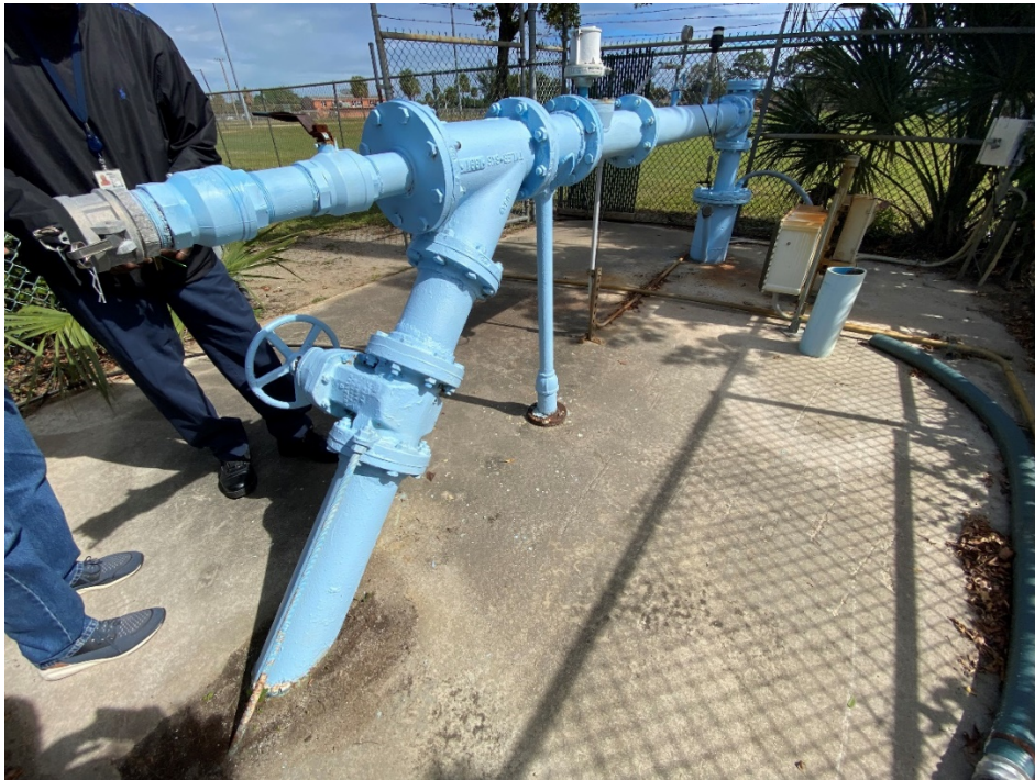
Figure 1. Well #14 Discharge Piping
